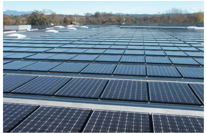
▲ Solar installation mounted parallel to the angle of the roof can mitigate wind effects.
