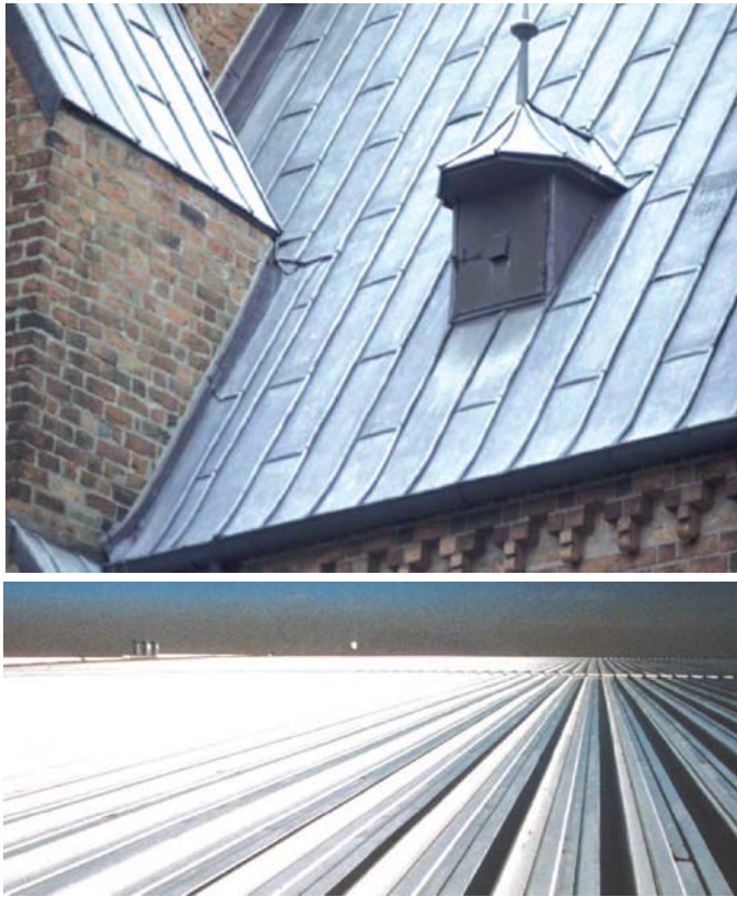
▲ In early days of metal roofing, pan lengths were short, so thermal movement never accumulated. As the “unbroken length” of panels increases, so does the dimensional gain or loss caused by surface temperatures.
