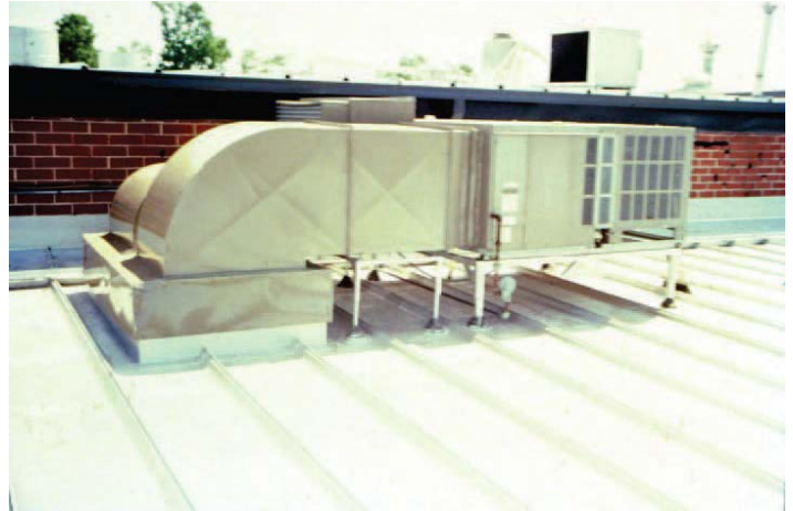
▲ This frame-mounted HVAC unit uses pipe supports that extend to the building structure and are flashed through the roof using rubber pipe flashings.
