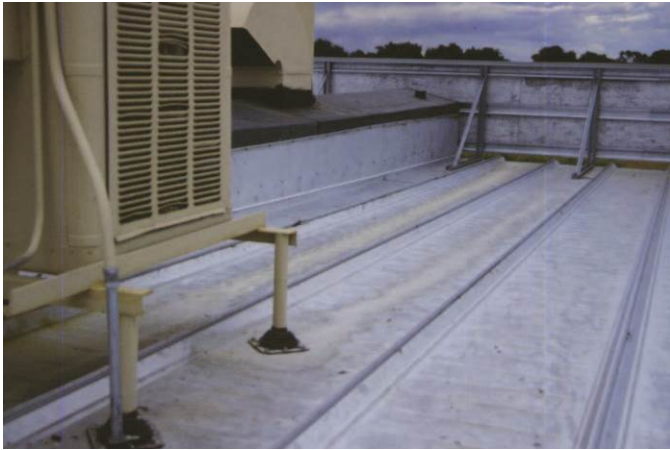
Drippage from a rooftop unit can cause corrosion as shown on this 1 ½-year-old roof. In another year and a half, the white zinc oxide trails will turn red with iron oxide.
