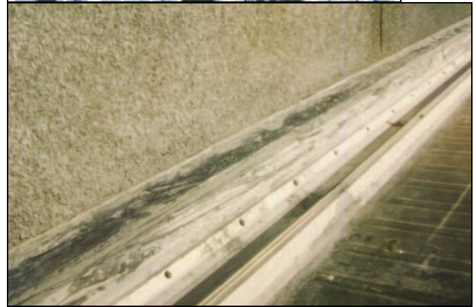
(Top) Improper storage and/or transit of Galvalume panels can result in damage from trapped moisture.
