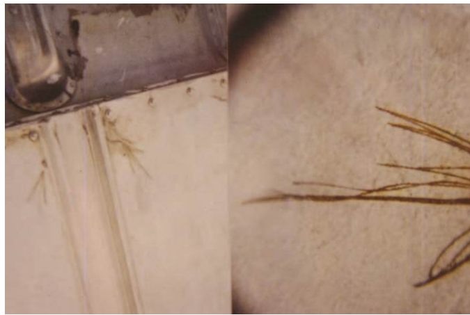
Markings from a punch listing by the installer are beginning to show traces of red rust.
