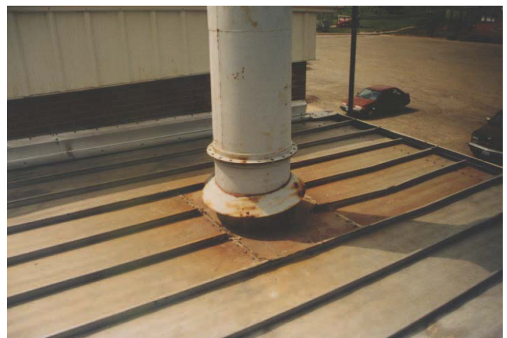
▲Exhaust flues that discharge gases from burning fossil fuels can cause a micro-acid rain environment near the flue.
